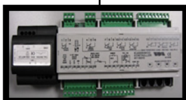
Micromaster Control Box Installed next to Room Fuse Box (out of sight)
